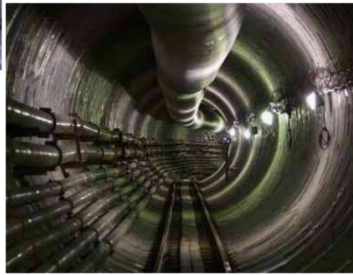
12" (300mm) & 14" (350mm) R-88 couplings used in tunnel boring / mining application. The pipe line delivered a bentonite water mixture while the outflow was an aggressive rock and mud slurry, Portland, Oregon, USA
